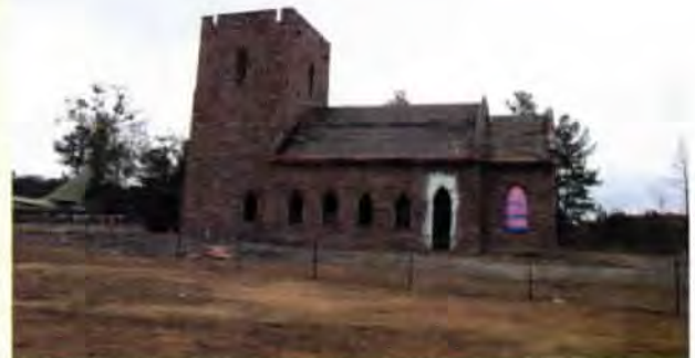
Chapel of The Fallen Eagles neaving completion in the Memorial Gardens at The Heritage Museum. Stained glass windows presently being installed
